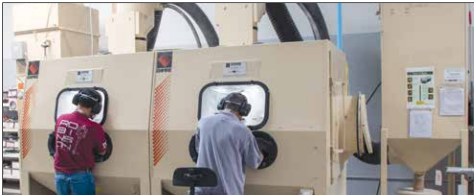
Media blasting room
